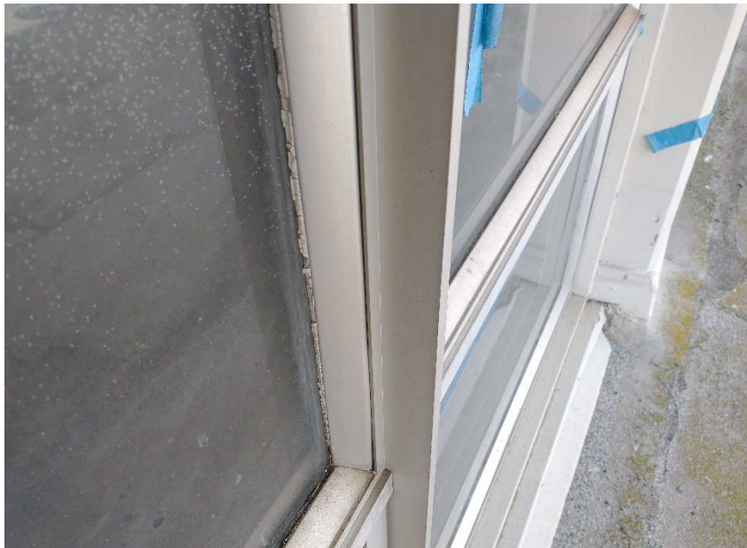
Window Frame Showing Glazing Putty
