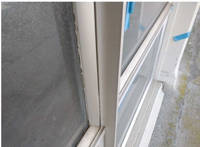
Window Frame Showing Glazing Putty
