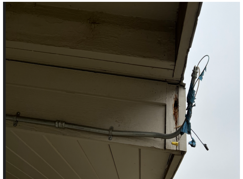
Open Electrical Conduit with Exposed Wires
