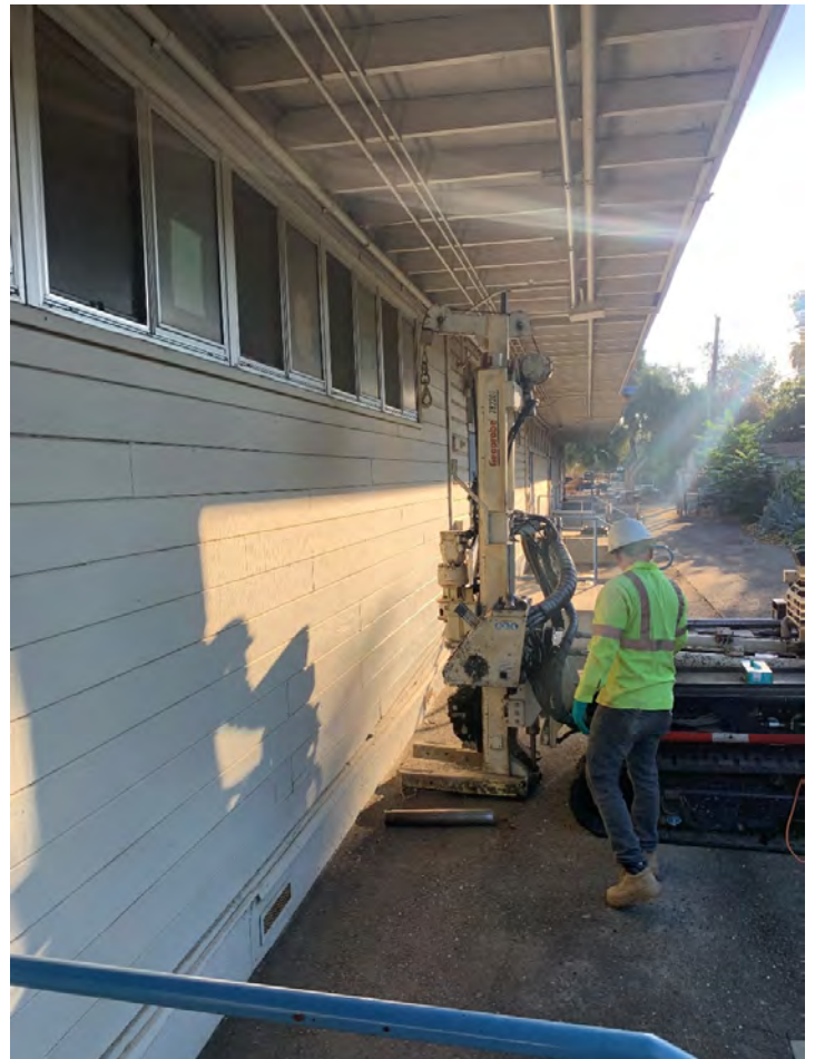
Photograph of Geoprobe drill rig obtaining soil sample from portable classrooms along south side of the school site
