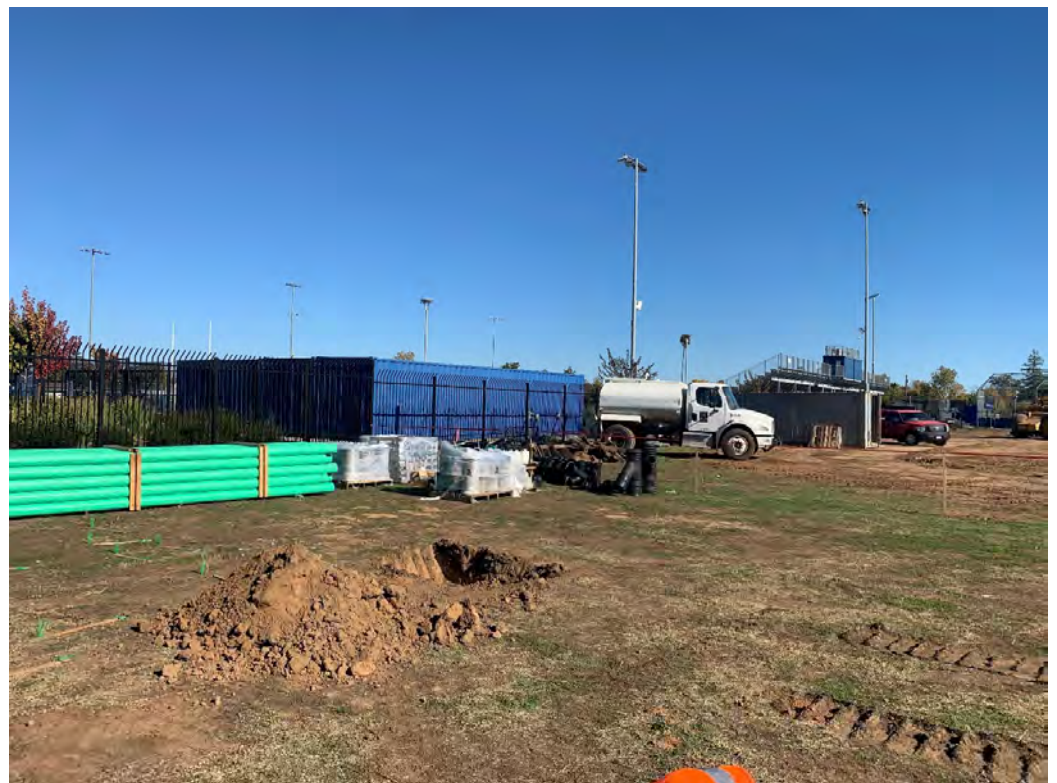
Final excavation depth and location of IDW action at B-56 with removal of lead-impacted soil prior to placement in drums.
