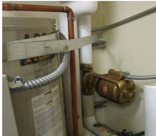
Water Efficiency No hot water at Science Lab sinks, hot water circulation pump appears to be seized. Recommend repair/replacement of pump.
