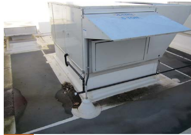
Energy & Atmosphere - Mechanical Many classrooms exhibit excessive AC unit noise. Further study is recommended.
