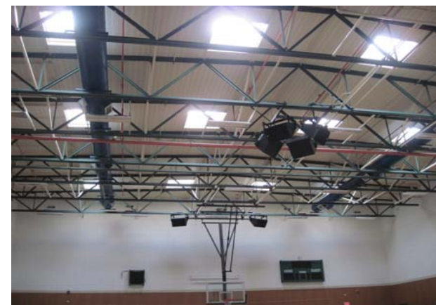
Indoor Environmental Quality Gym lighting is not multi-level control, which is required by T24. No automatic day lighting control in spaces with ample natural light (gym skylights).
