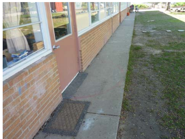
Materials & Resources Interior Drainage issues include sidewalk slopes into the building, resulting in doors will not fully close.
