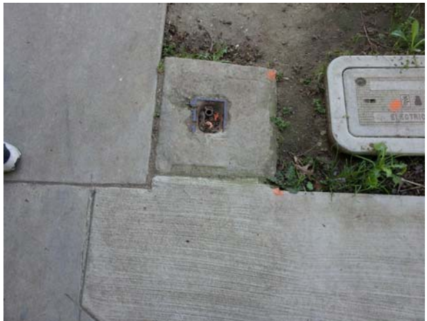
Water Efficiency Exterior Existing hose bib is at grade, filled with dirt and should not be used without back flow prevention.
