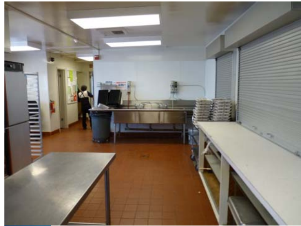
Water Efficiency Interior Waste from the food wash sink has a direct sewer connection. This should have indirect connection.
