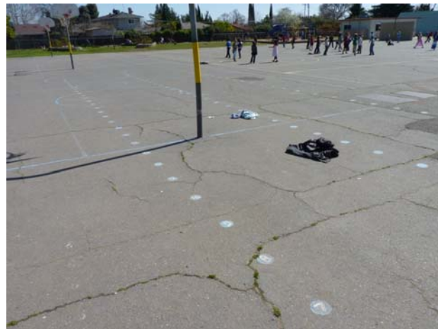
Sustainable Sites Outdoor Activity Play surface is uneven and cracking, needs repair, slurry seal and re-striping.
