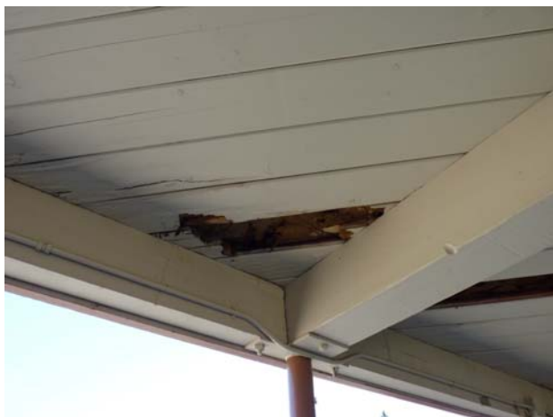
Materials & Resources Exterior Water ponding on roof is contributing to the dry rot of the roofing structure.
