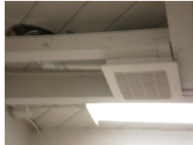
Energy & Atmosphere Restrooms are not conditioned. They are only exhausted by dedicated ceiling exhaust fans.
