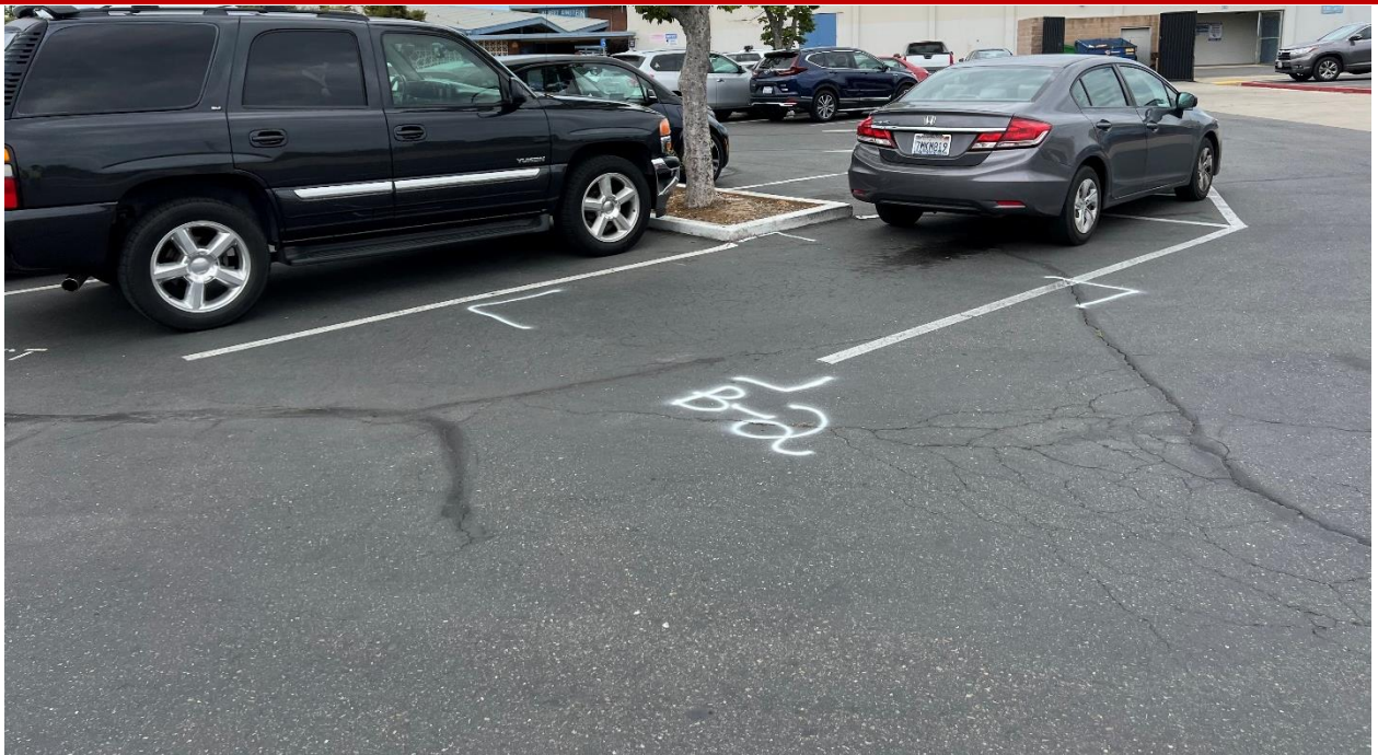
Longitudinal, transverse, and alligator cracking near boring B-2
