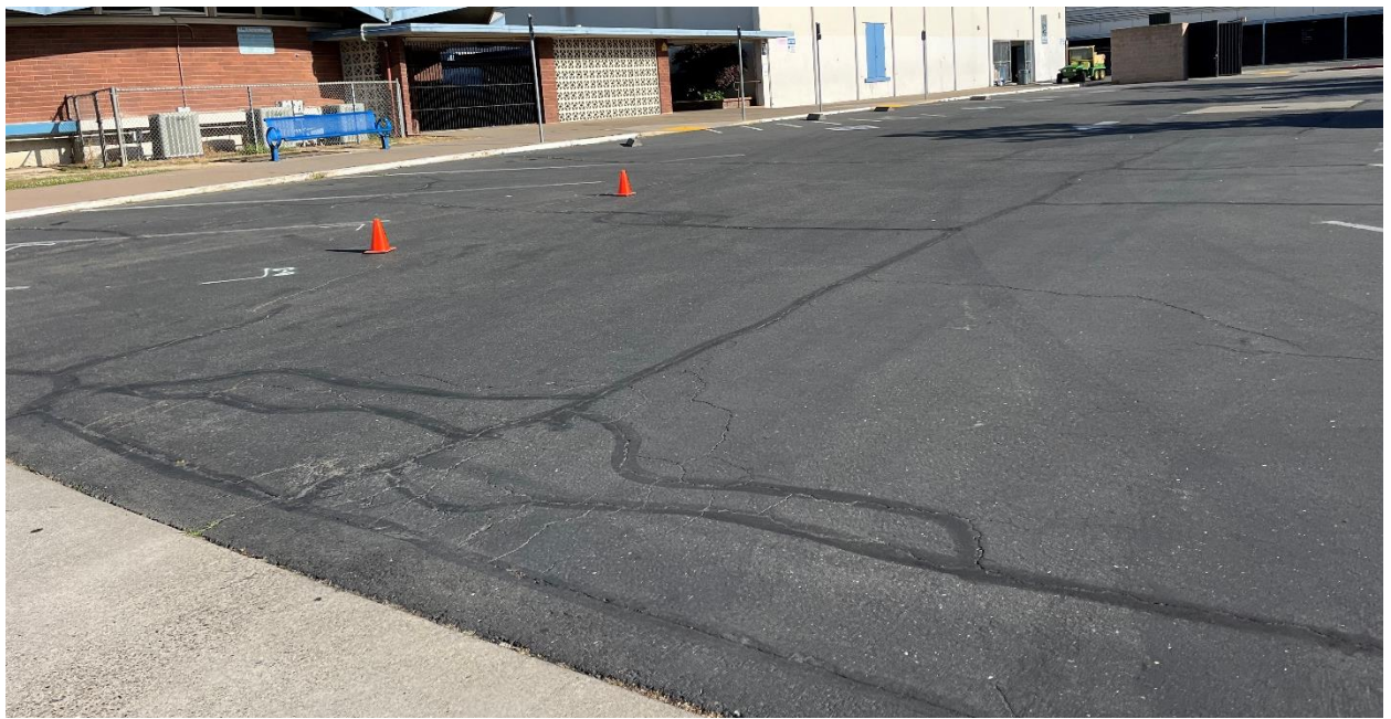
Longitudinal, transverse, and alligator cracking near boring B-5
