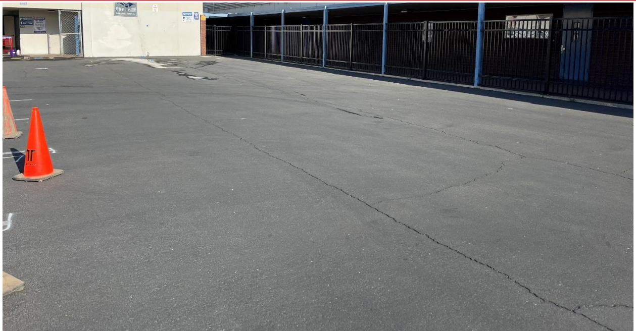
Longitudinal and transverse cracking near boring B-1
