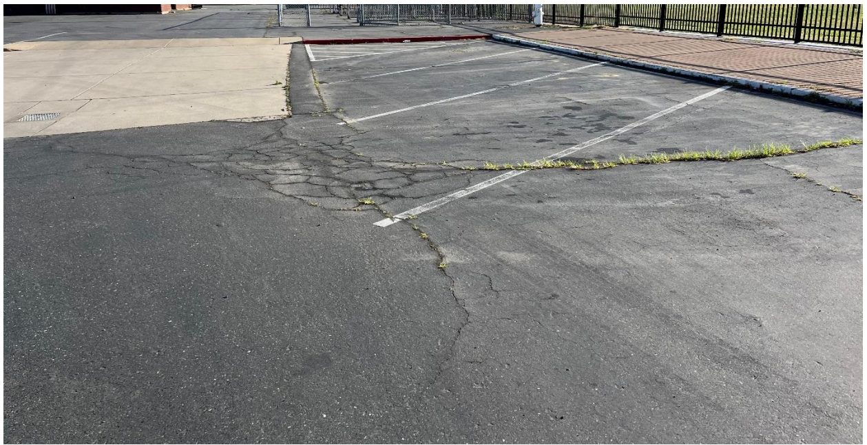
Longitudinal, transverse, and alligator cracking near boring B-2
