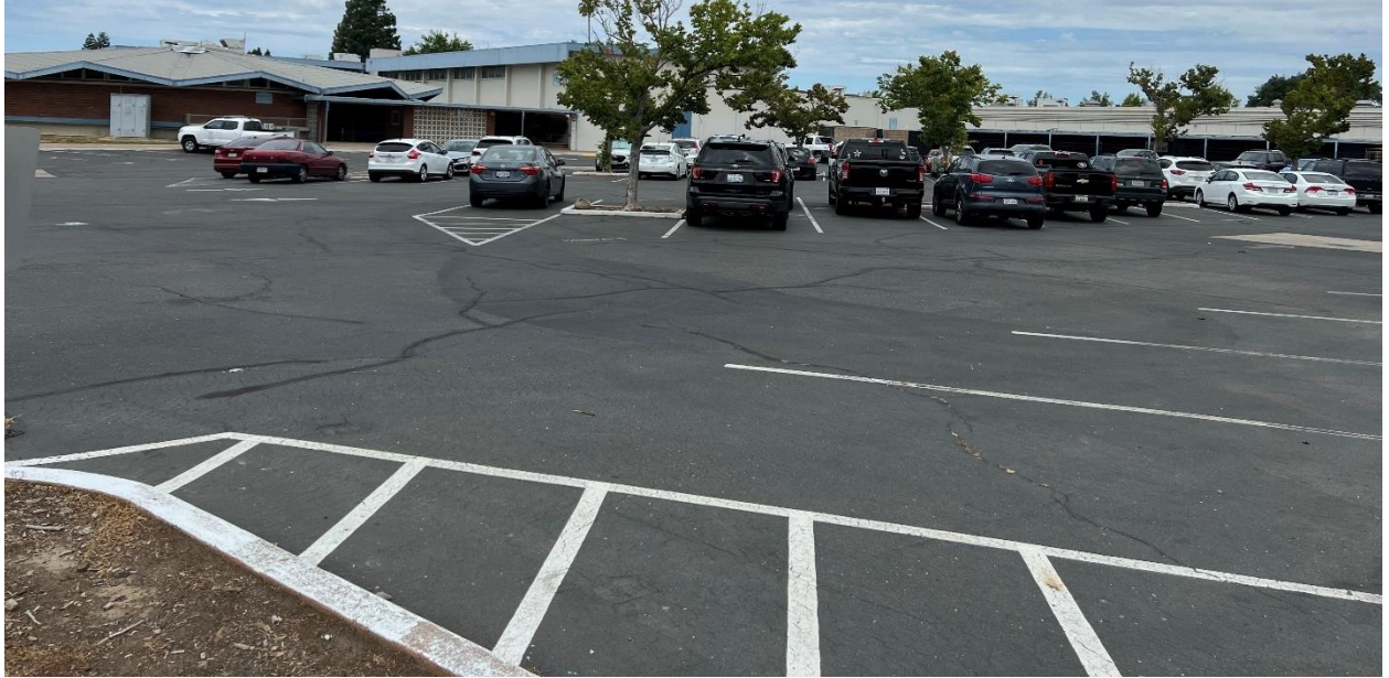
Longitudinal and transverse cracking between borings B-4 and B-6
