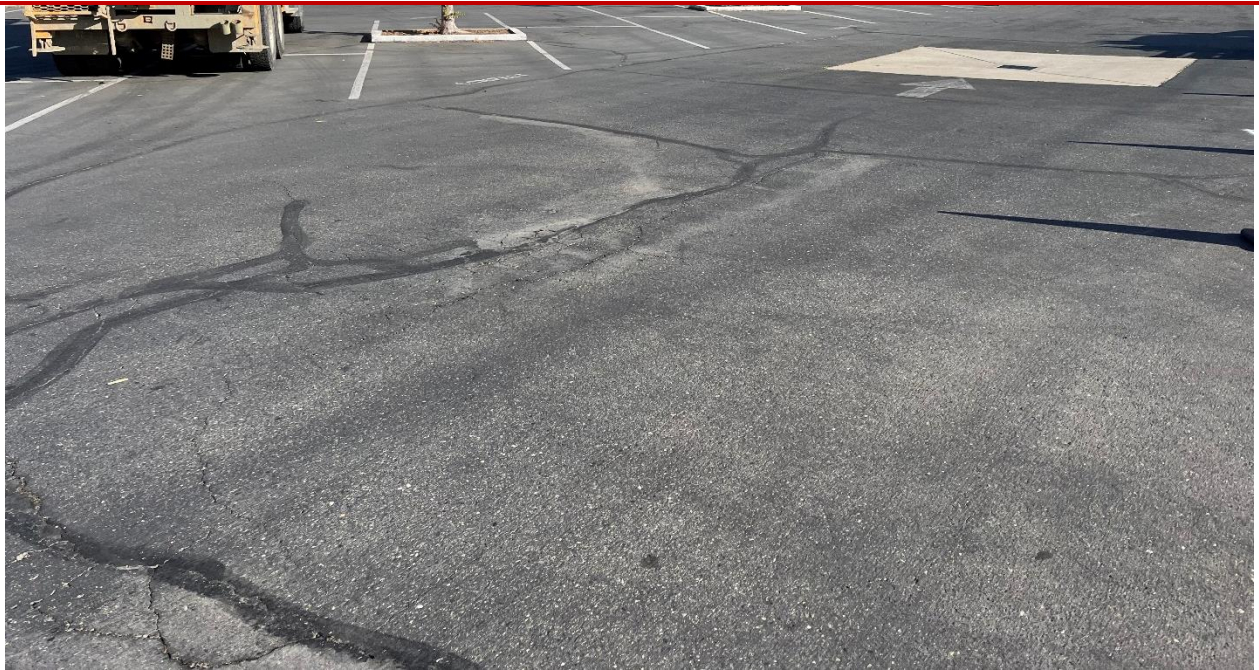
Longitudinal, transverse, and alligator cracking near boring B-4
