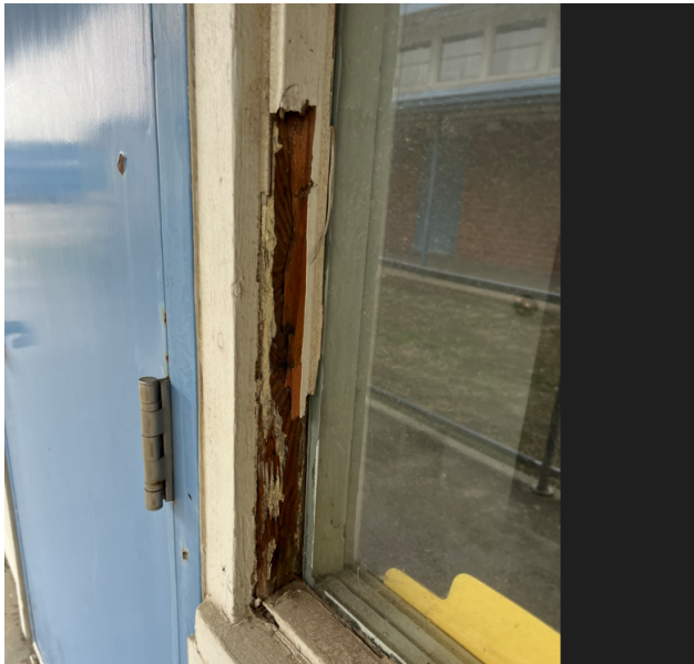
Dry Rot at Side of Window
