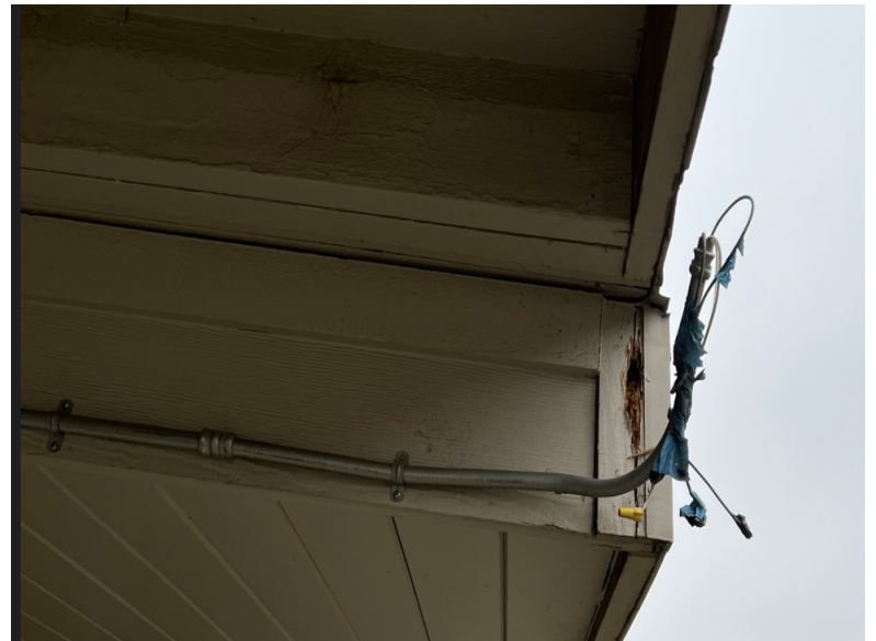
Open Electrical Conduit with Exposed Wires
